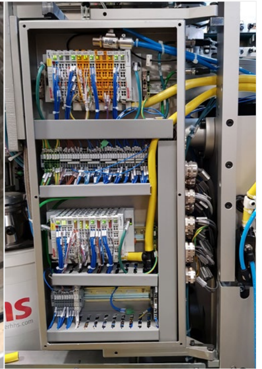
Cooling of control cabinets
